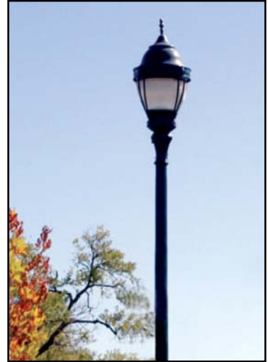
Pedestrian level lighting
