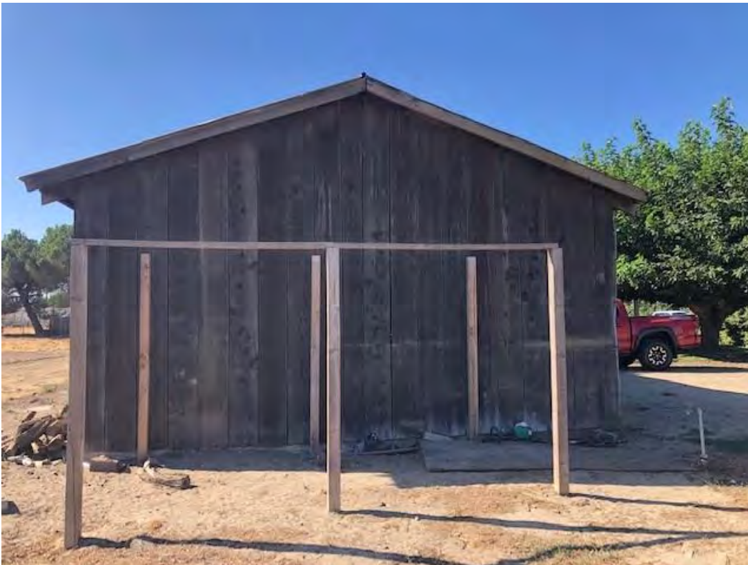
O) View looking south of the north facing façade of Building No. 3. 8/31/2021. Acc. # 21-3598.
