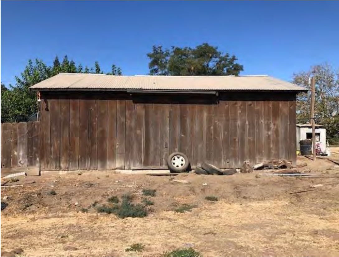
L) View looking west of the east facing façade of Building No. 3. 8/31/2021. Acc. #21-3597.
