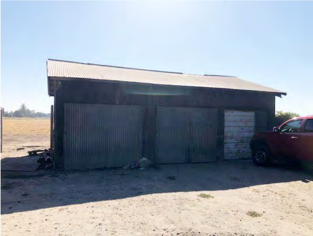
N) View looking east of the west facing façade of Building No. 3. 8/31/2021. Acc. #21-3601.
