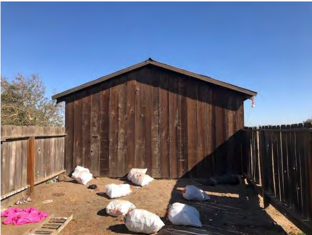
M) View looking north of the south facing façade of Building No. 3. 8/31/2021. Acc. # 21-3596.
