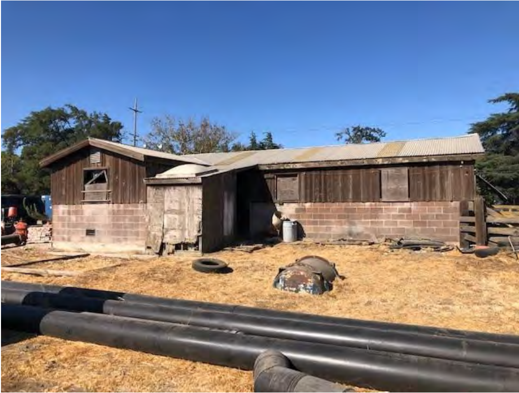
I) View looking west of the east facing façade of Building No. 1. 8/31/2021. Acc. #21-3604.
