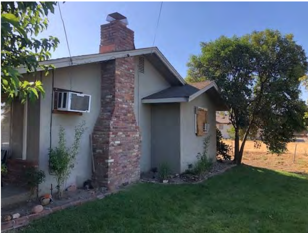
B) View looking southeast of the west facing façade of the residence. 8/31/2021. Acc. # 21-3590.
