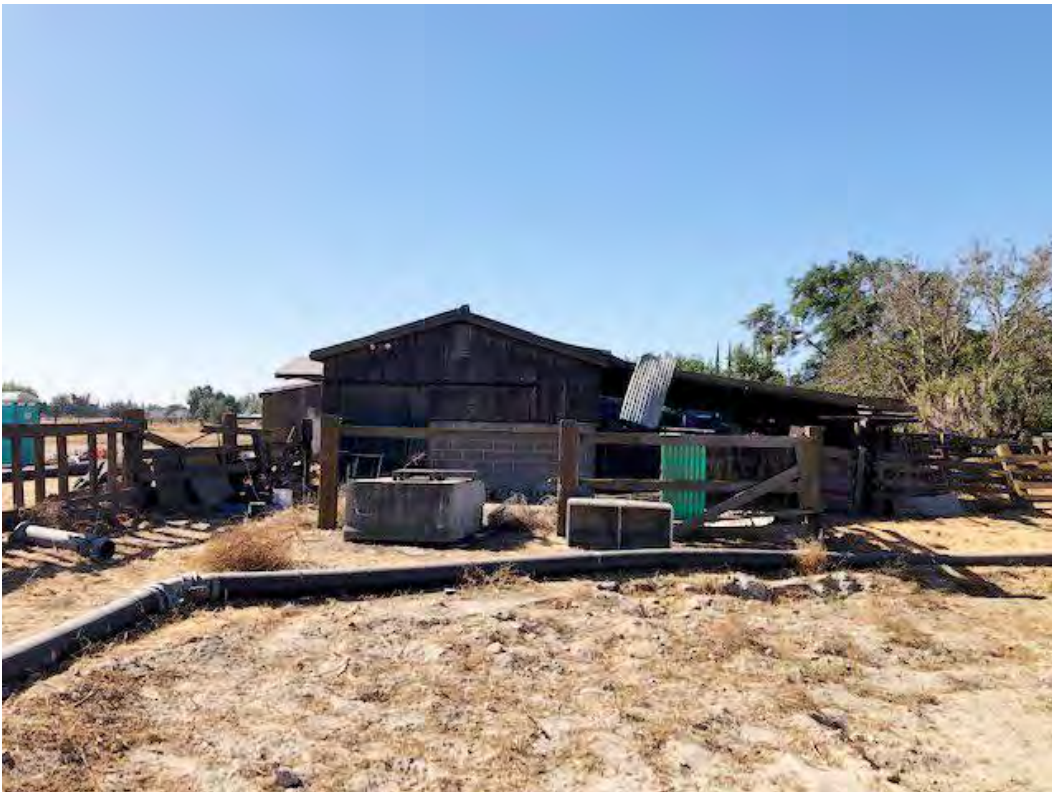
J) View looking south of the north facing façade of Building No. 1. 8/31/2021. Acc. # 21-3609.
