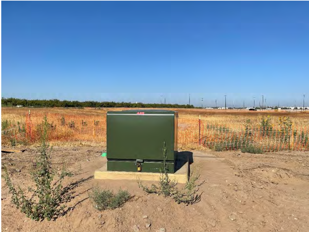
Photograph 11: View of transformer along eastern property boundary (looking west).
