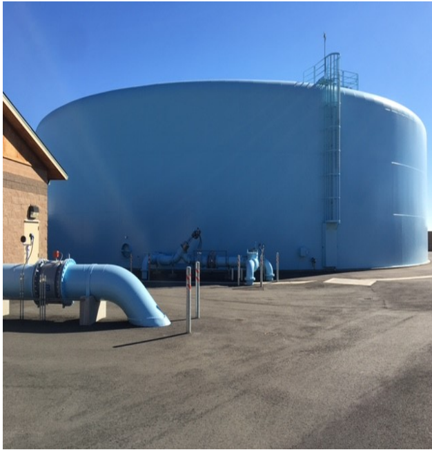
Atherton Drive Storage Tank and Booster Pump Station. Five variable frequency pumps, onsite treatment, and a 3.7 million gallon tank serve peak water demands. The facility was completed in 2014.
