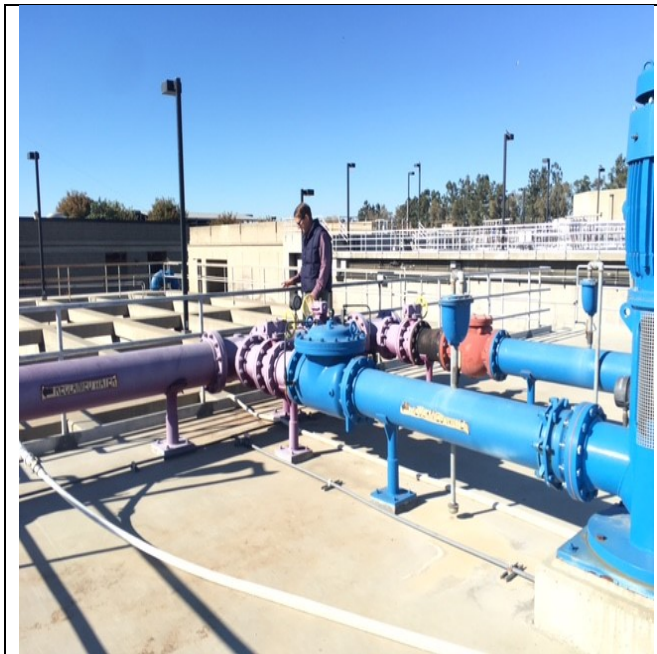
Recycled water is diverted for construction dust control at the Wastewater Quality Control Facility.
