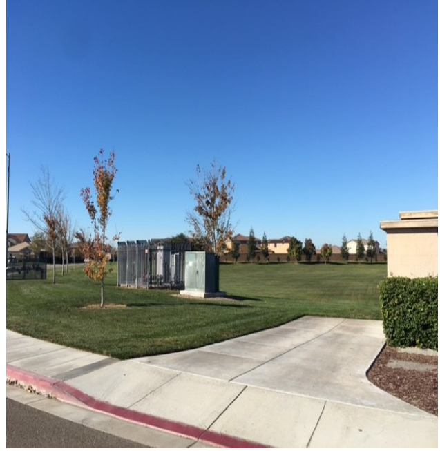
An irrigation well and stormwater pump station are both located at Tesoro Park on Tesoro Drive
