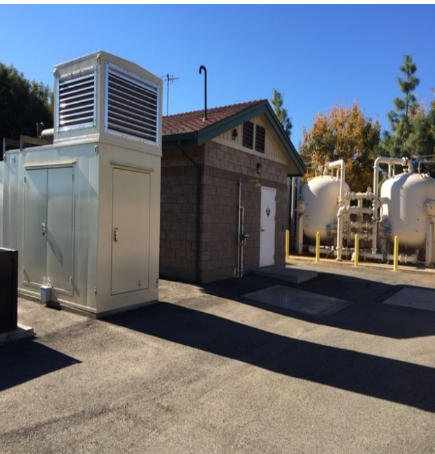
Well 24, off of Van Ryn Avenue, is one of several City wells with onsite manganese green sand filtration to remove arsenic, which is a problem at deeper levels of the aquifer.
