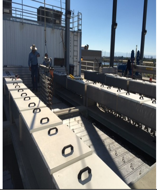
Wastewater Quality Control Facility ultraviolet contact chamber, during servicing of the ultraviolet bulbs.
