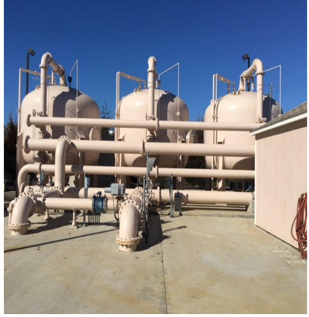
Wells 13, 19, and 21 have local treatment facilities for arsenic removal, but nitrate, manganese, and TCP 123 are treated at a central treatment facility, shown above, where blending with surface water is performed.
